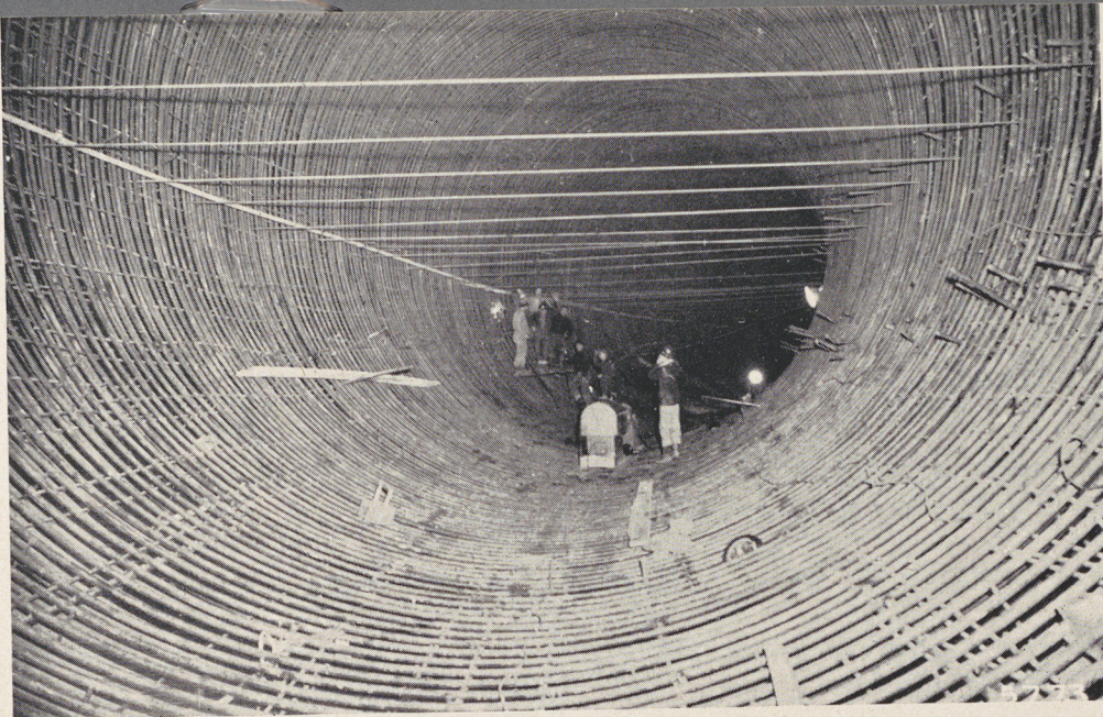
In the tunnel built to divert the Eucumbene River while the Adaminaby Dam is being constructed. Reinforcing steel is in position for the concrete lining.
