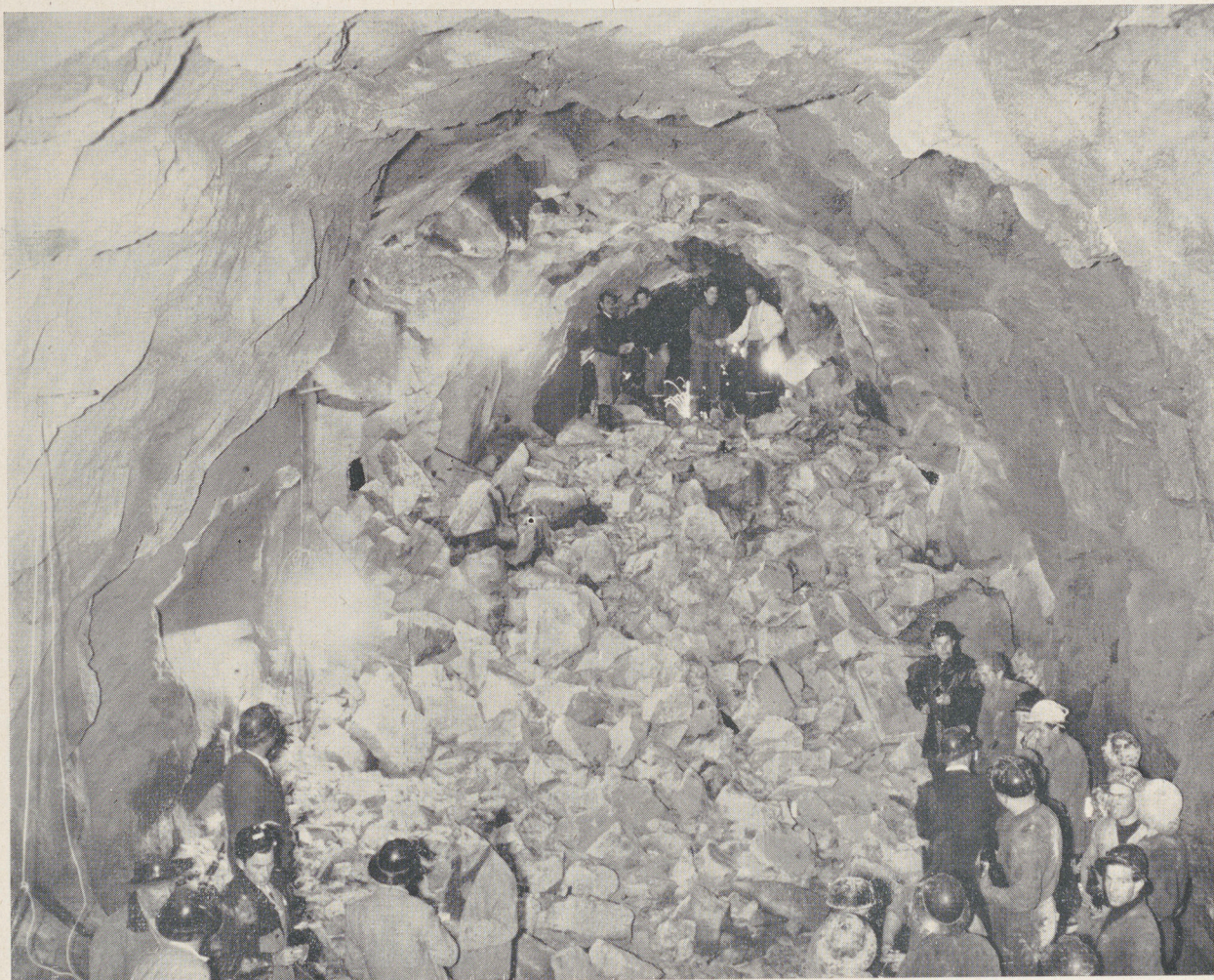
Tunnelling is speeded up by working from both ends, and from intermediate points as well wherever practicable. Here is the final break-through in the Guthega tunnel.
