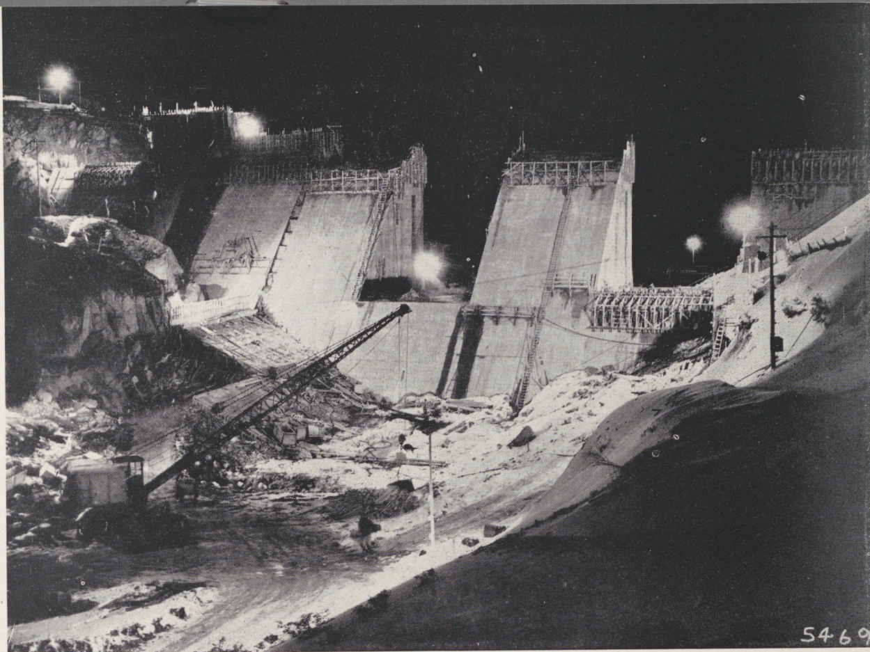
Work on the major projects of the Scheme continues day and night. This is a night scene during the building of Guthega Dam, at the junction of the Snowy and Guthega Rivers.
