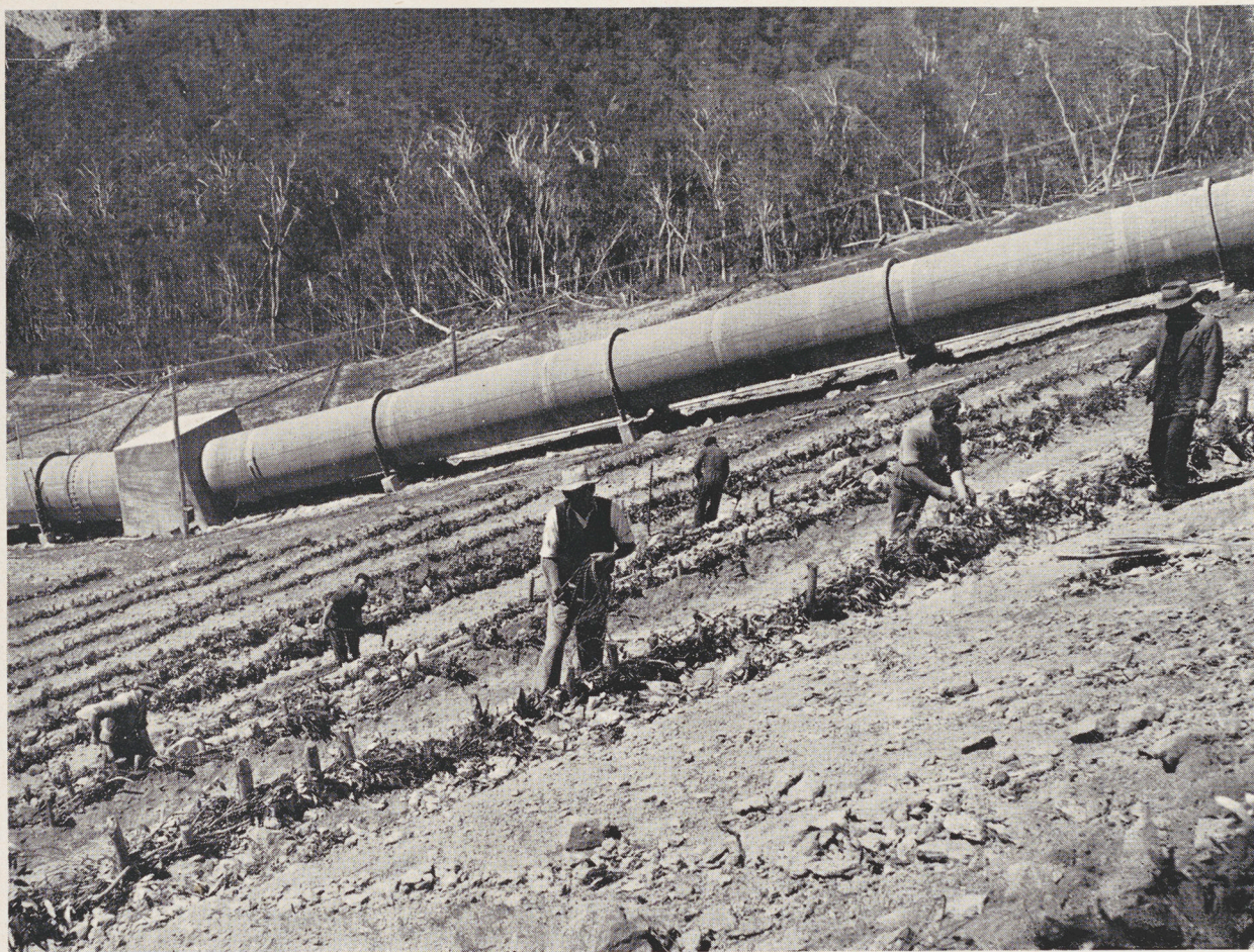
Soil conservation protective work adjoining Guthega penstocks. The Authority has given special attention to the prevention and repair of soil erosion arising from engineering works.
